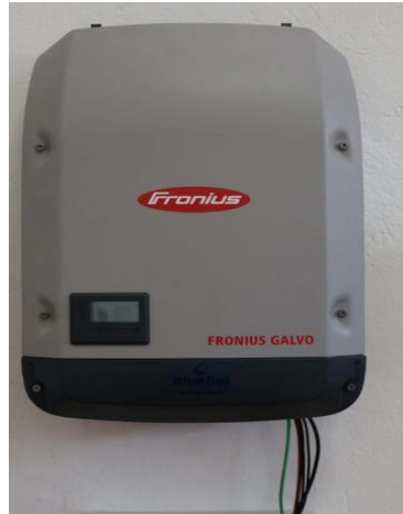
Figura 10: Inversor Solar Fronius
